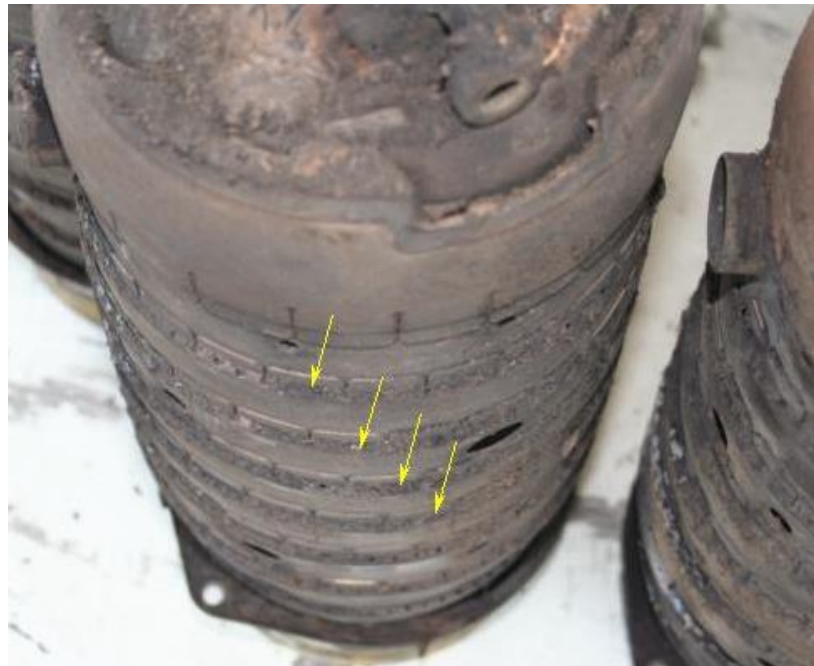
Figure 14: No. 1 engine burner cans exhibited deposited debris on high spots (largest diameters)
