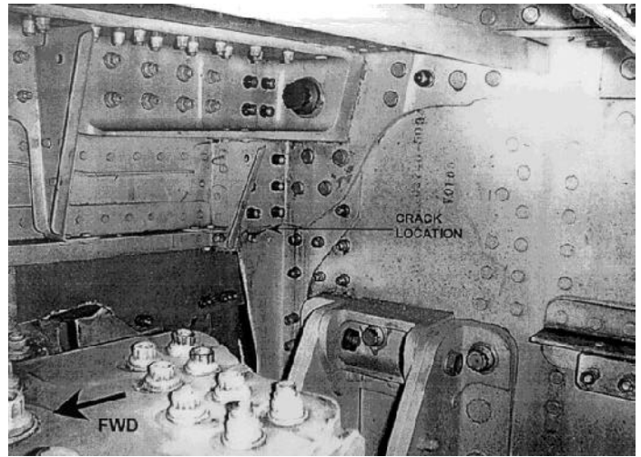
Figure 3: Fatigue crack in an Ansett B-767 body station 1809.5 bulkhead outer chord.
