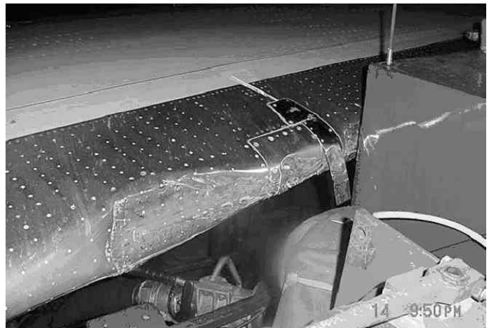
Figure 2: Detailed view of the damage with fuel truck.
