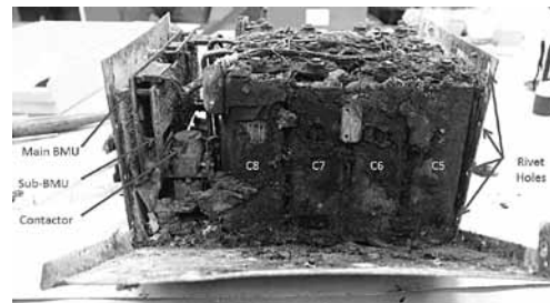
Figure 6: View of battery with battery case panel pulled back to reveal cells 5 through 8.
