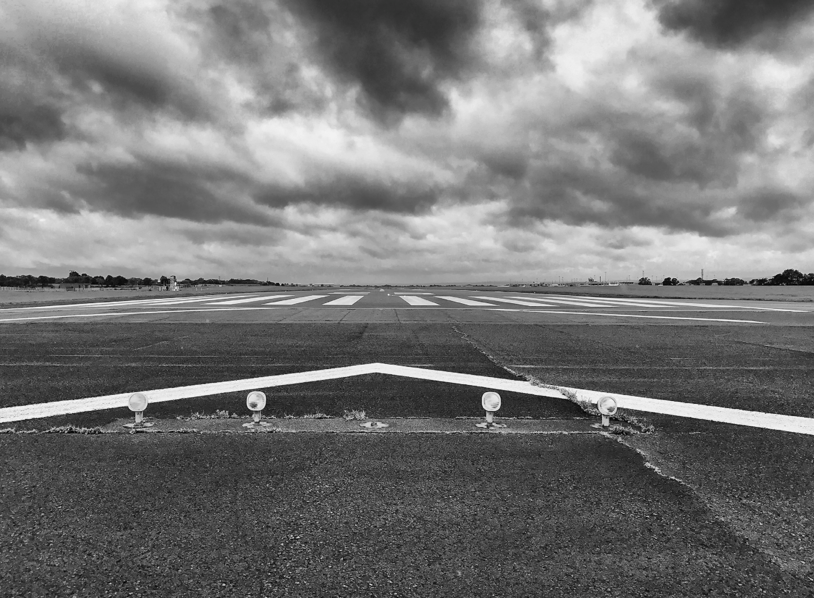
Figure 1. The damaged approach light.
